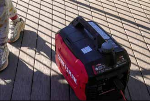
Kaylin Johnson, whose home is one of the few that survived the Eaton Fire in her neighborhood in Altadena, Calif., walks past a generator running to provide power at her home.
